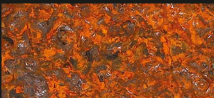
Without corrosion protection treatment
